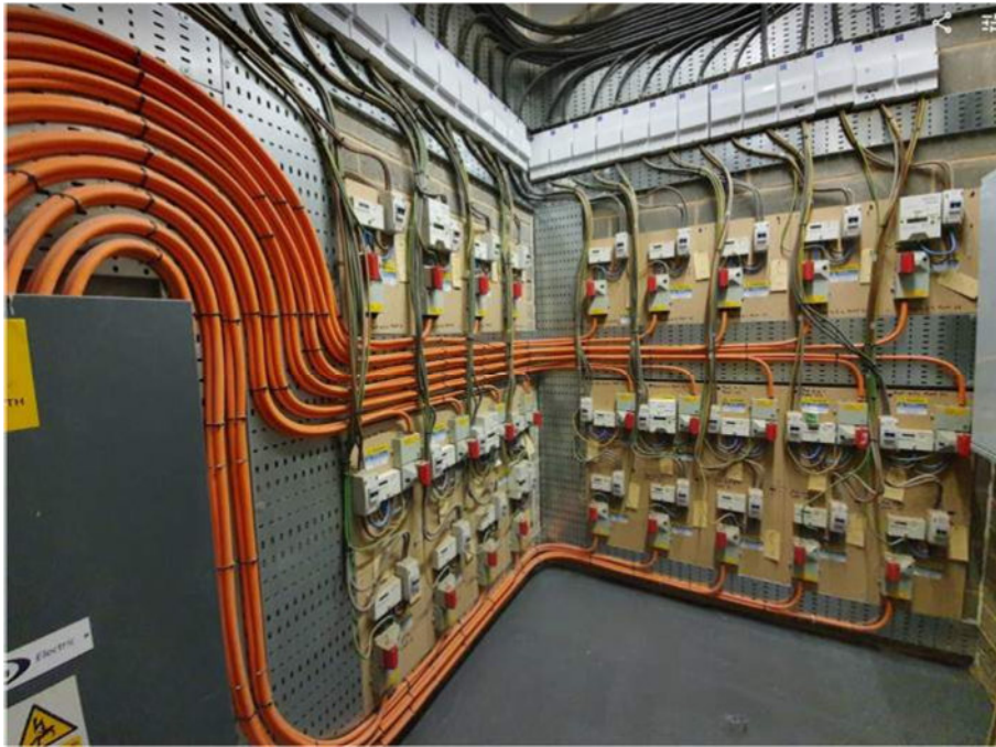
Separate plantroom with Block 4 meters in the basement.
