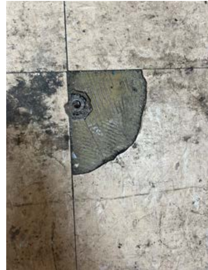
Views of asbestos containing materials found on site within the existing, on-site, 1-2No. storey building.
