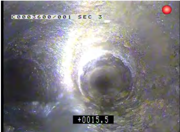
GULLYX_cfbfb68-e0be-425c-a01d-3d8438f830c9_20170824_131121_822.jpg, 00:02:34, 15.50m Junction at 9 o'clock, diameter: 100mm
