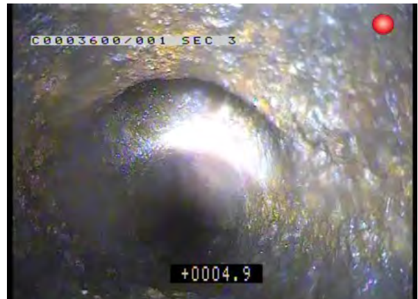
GULLYX_e6cea38e-25f1-4658-9ebd-6f6ab1a0be2d_20170824_130911_648.jpg, 00:01:30, 4.90m Junction at 12 o'clock, diameter: 100mm
