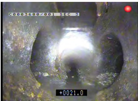
GULLYX_2dd90ab7-53dd-4902-8b93-1cdd8c3dc74b_20170824_131228_540.jpg, 00:03:09, 21.00m Junction at 3 o'clock, diameter: 100mm
