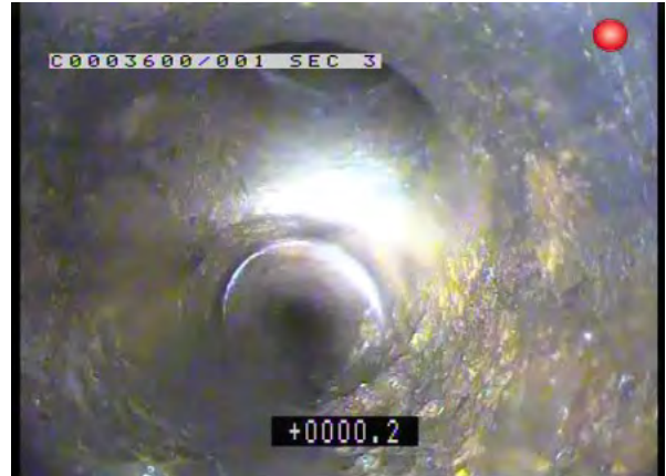
GULLYX_8b33ade3-fc07-4751-89fa-16827cc054ba_20170824_130805_937.jpg, 00:01:00, 0.20m Junction at 12 o'clock, diameter: 100mm
