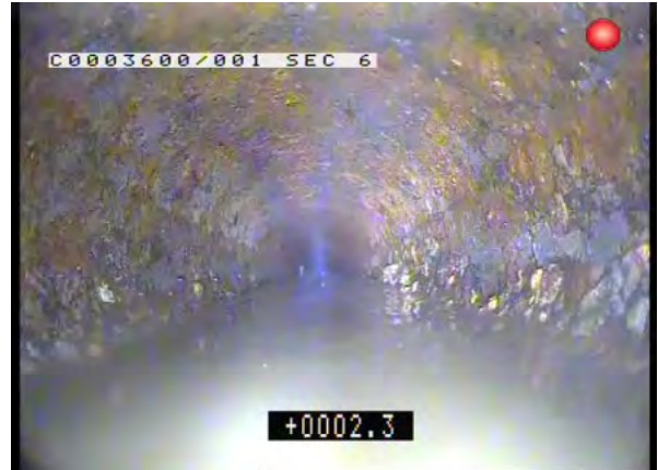
SW1X_4aa6789e-51c5-47d0-b167-90124c401110_20170824_132143_642.jpg, 00:00:20, 2.30m Water level, 10% of the vertical dimension
