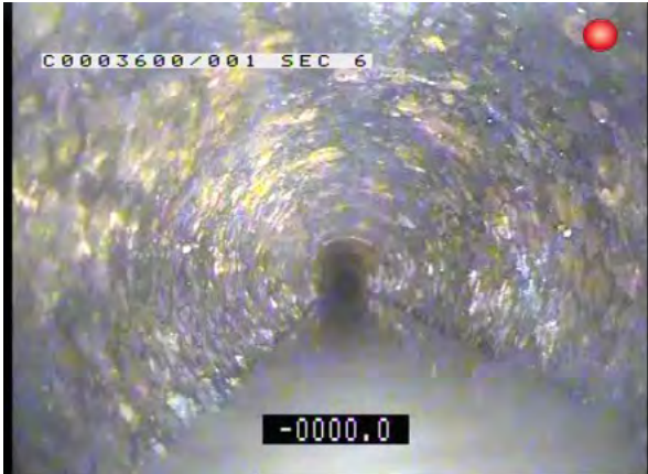
SW1X_42f3eab4-fc1b-403f-9e39-5eda5f1000fc_20170824_131948_443.jpg, 00:00:00, 0.00m Start node type, manhole, reference number: SW1
