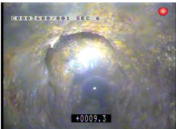
SW1X_243a8409-1834-4bc0-be0e-16071e3a554e_20170824_132307_211.jpg, 00:00:54, 9.30m Junction at 11 o'clock, diameter: 100mm
