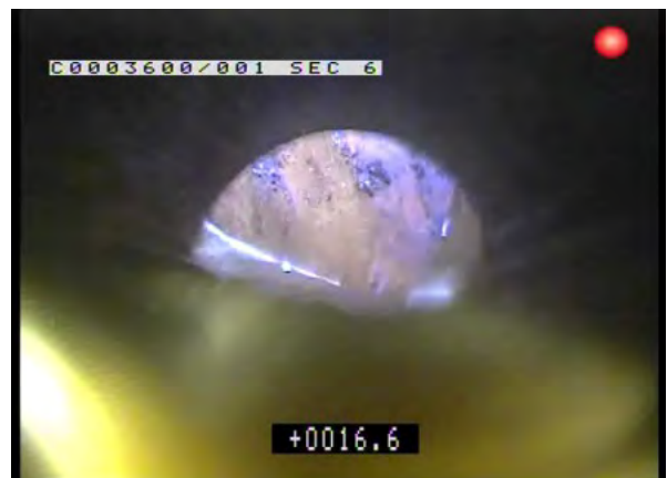
SW1X_a9807cbf-935b-4227-93ae-bbb2dcf80117_20170824_132504_659.jpg, 00:02:02, 16.60m Finish node type, manhole, reference number: SW2
