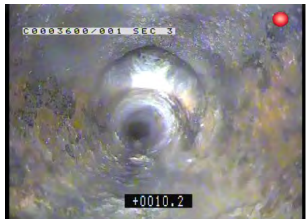
GULLYX_1032c5f9-15bc-46af-bc6e-35cdb97d10b2_20170824_131026_437.jpg, 00:02:00, 10.20m Junction at 12 o'clock, diameter: 100mm
