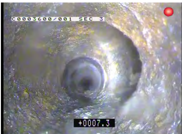
GULLYX_2d001cc5-c8bf-4880-9be3-b9503964a490_20170824_130941_471.jpg, 00:01:40, 7.30m Junction at 3 o'clock, diameter: 100mm
