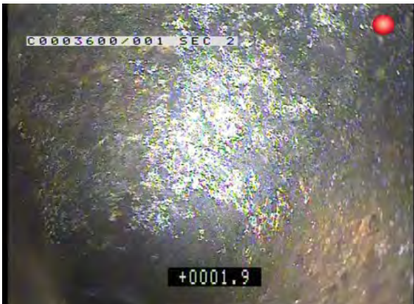
RWG2X_e89098c4-1efe-4dc8-80f4-da86b229d413_20170824_130330_347.jpg, 00:00:42, 1.90m Line deviates down
