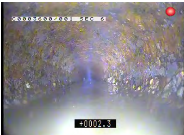
SW1X_08cef109-c8c3-4d99-b512-d535b8a4b1ca_20170824_132702_478.jpg, 00:00:20, 2.30m Surface damage, corrosion products from 4 o'clock to 8 o'clock,
