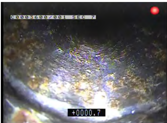
RWPX_b90c3937-81da-43ee-9148-c78e6cd11ce0_20170824_132949_775.jpg, , 0.70m Finish node type, gully, reference number: RWP
