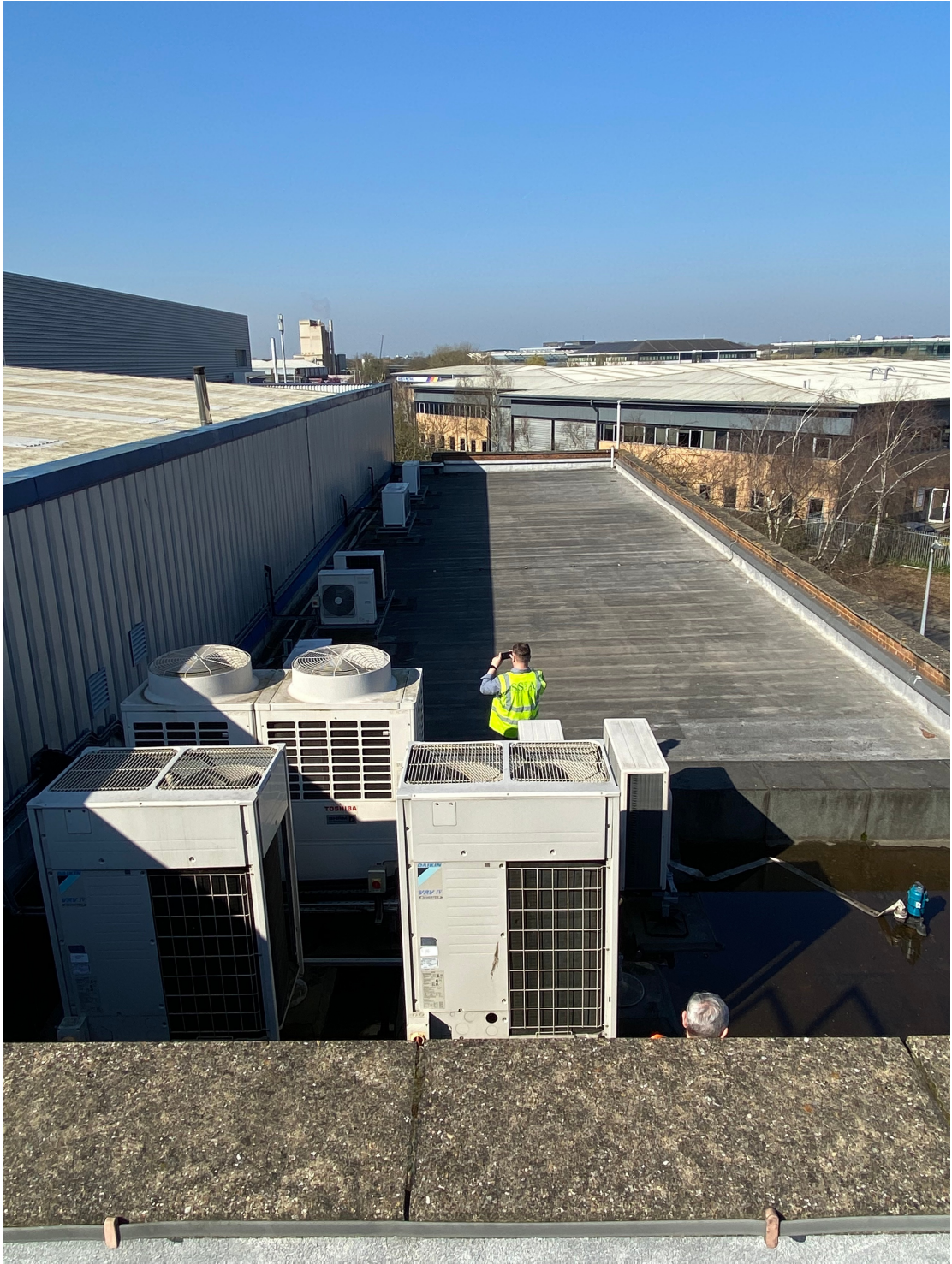
Existing air conditioning units on the office roof to be removed
