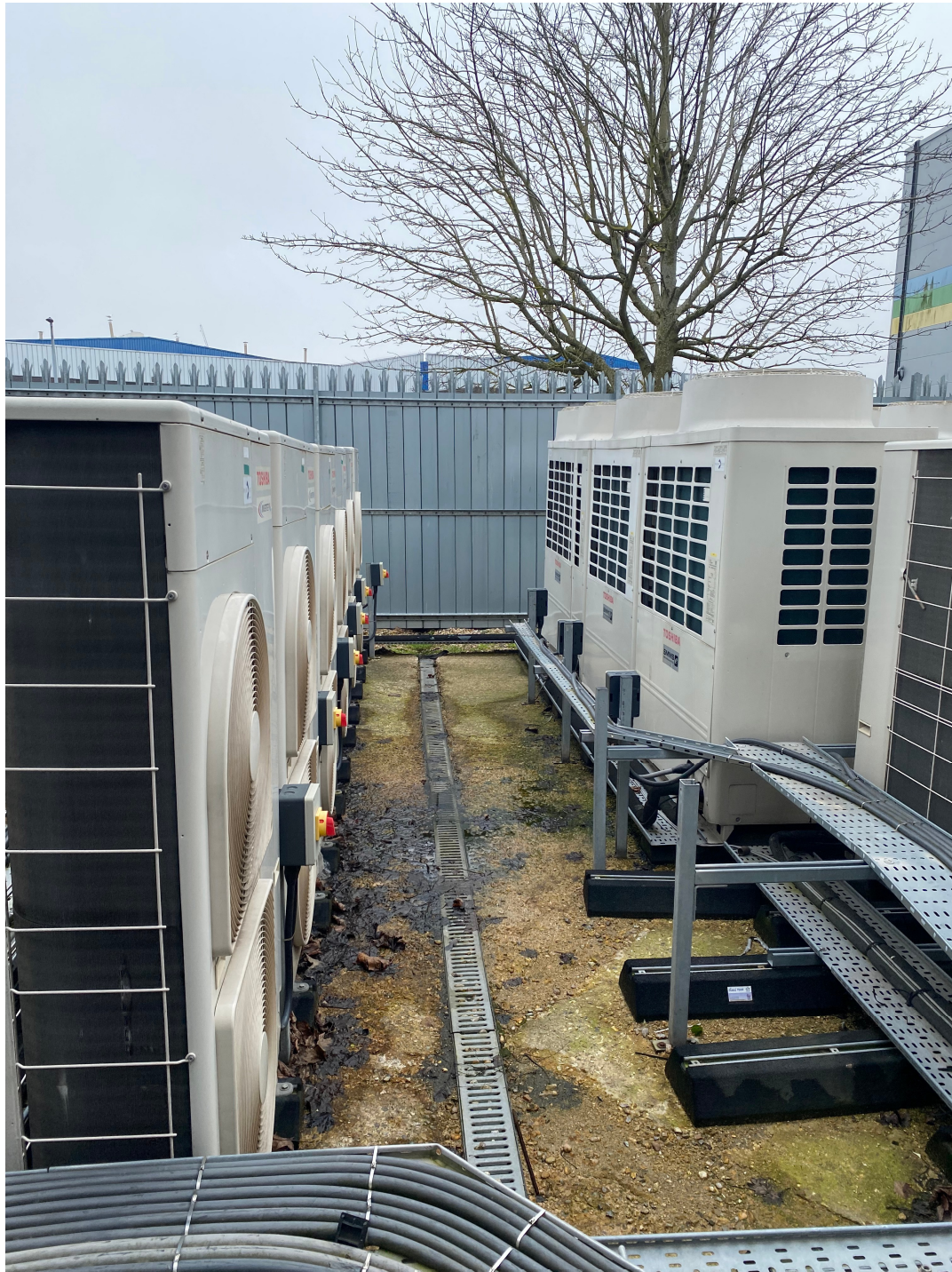
Existing air conditioning units within the Service Yard area to be removed
