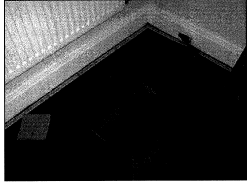
Bedroom, Room ID G05, Floor Intrusion (No Suspected Materials Seen)
