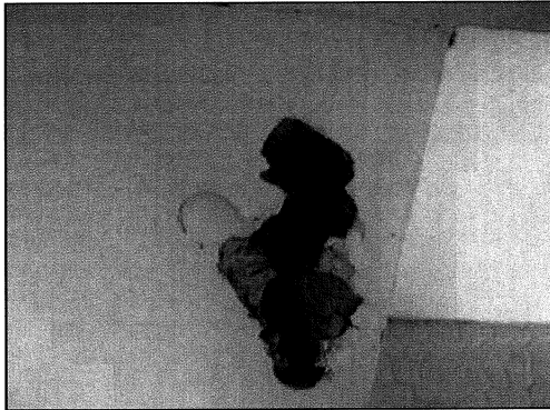
Bedroom , Room ID G05, Wall Intrusion (No Suspected Materials Seen)
