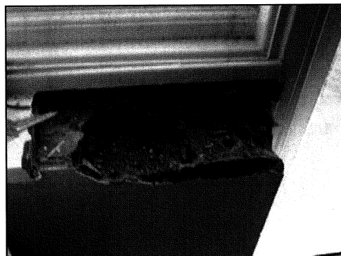
Bedroom, Room ID G04, Wall Intrusion (No Suspected Materials Seen)
