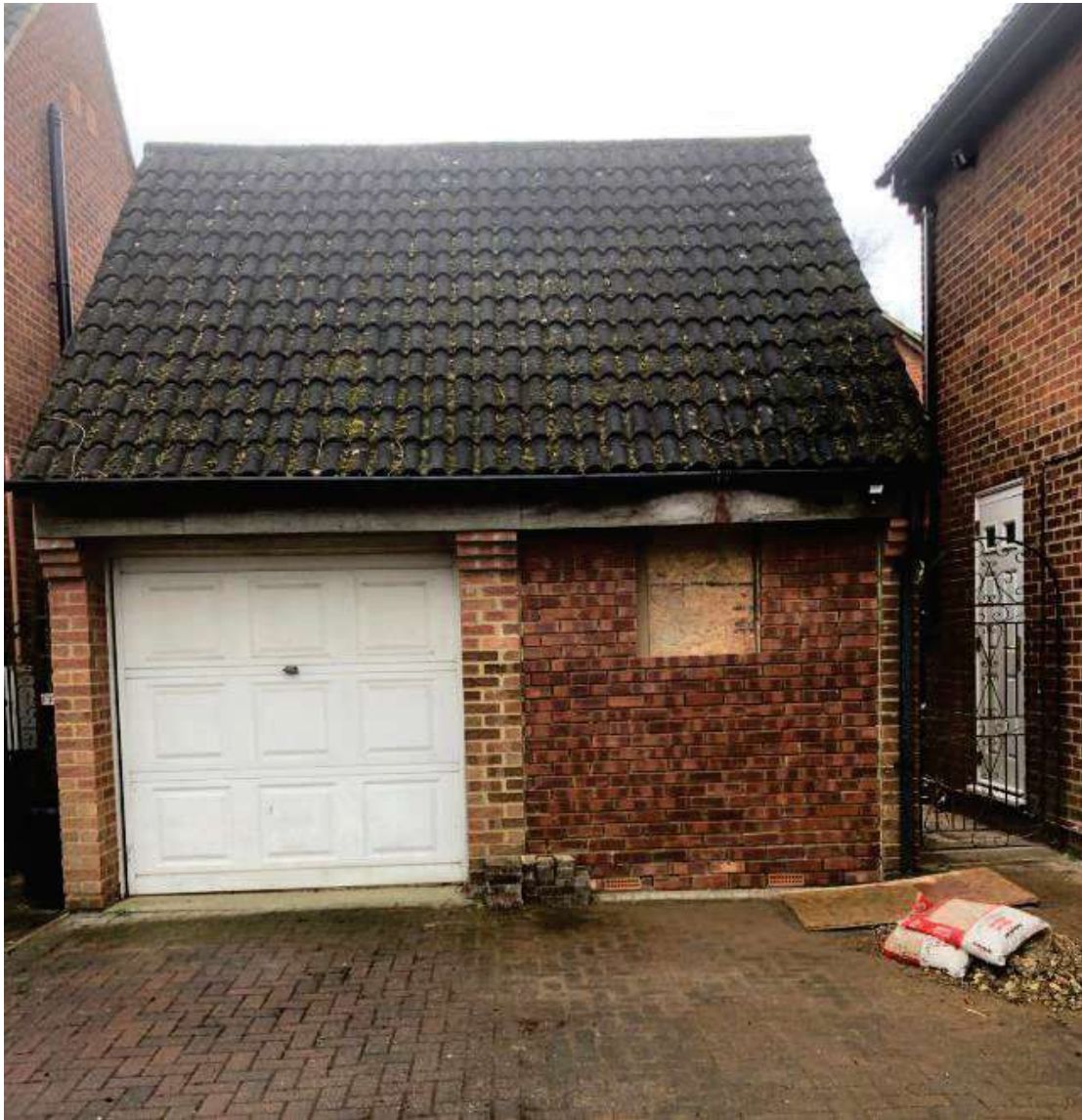
Figure 4: Photograph of Rear Elevation of Property and Relationship to 7 Pastures Mead on Right Side of Image
