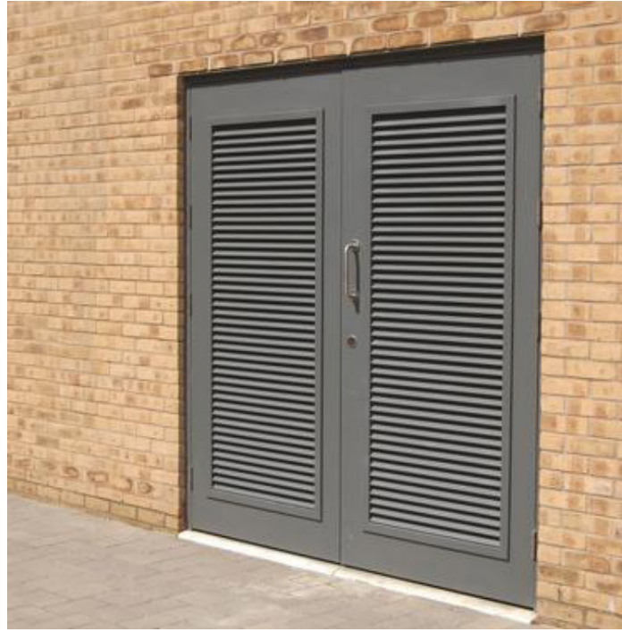
[13] Aluminium louvred plant door
