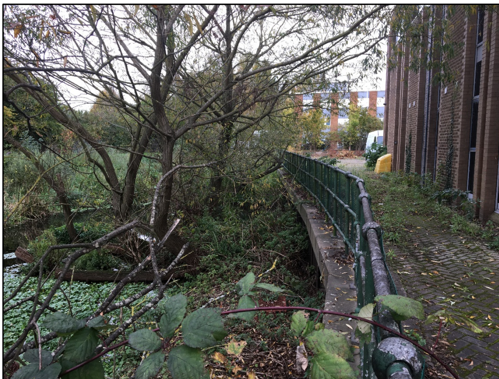
Photo of T3 & T4 growing at the bottom of retaining wall
