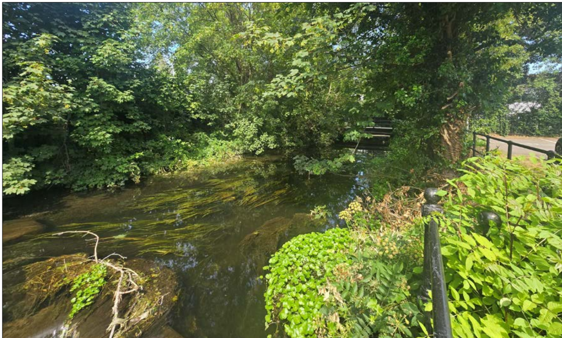
Figure 2 Trees growing adjacent to retaining wall
