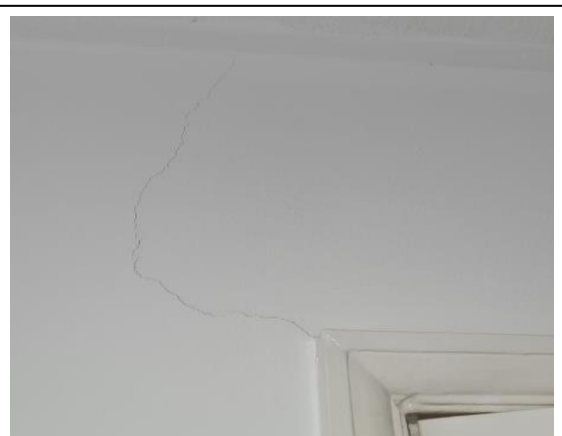
Photo 13: Flat 19 – Front Right Lounge- Cracking above door
