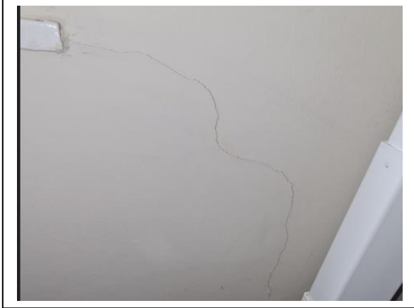
Photo 14: Flat 19 – Front Left Bedroom- Cracking below window
