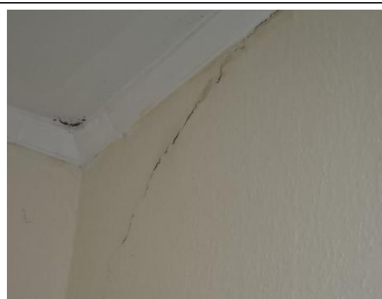
Photo 5: Flat 20 – Stairs - Cracking to Left Elevation
