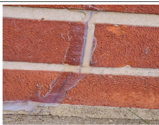
Photo 17: Front Elevation – Cracking below Ground Floor Left Window- Note evidence of previous repairs
