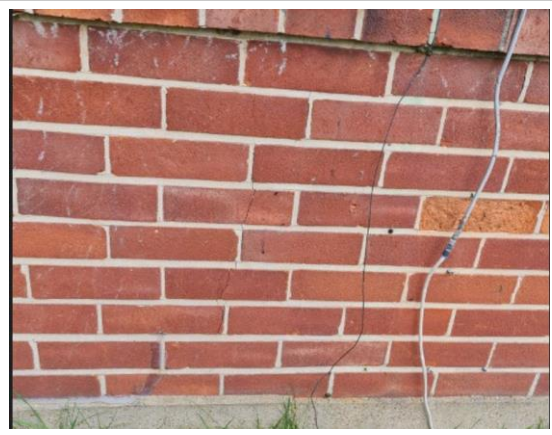
Photo 15: Front Elevation – Cracking below Ground Floor Left Window
