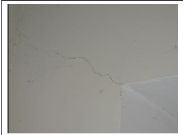
Photo 8: Flat 20 – Bathroom - Cracking Above LHS of Window
