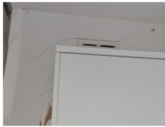
Photo 3: Flat 20 – Kitchen - Cracking to Left Elevation
