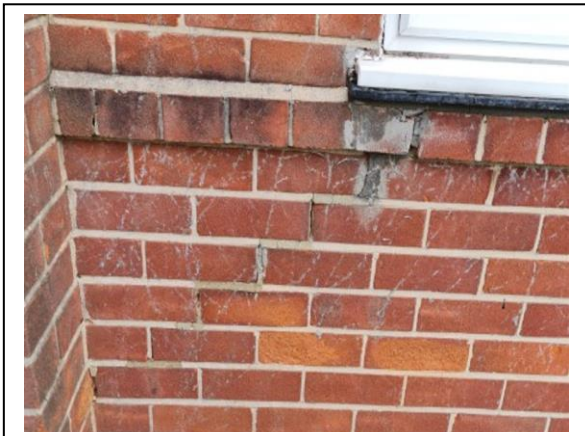
Photo 16: Front Elevation – Cracking below Ground Floor Left Window- Note evidence of previous repairs
