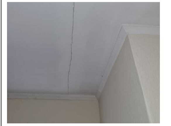
Photo 6: Flat 20 – Landing - Cracking to Ceiling
