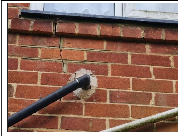
Photo 20: Rear Elevation – Cracking below First Floor Middle Window- Note evidence of previous repairs & possible presence of Helibars
