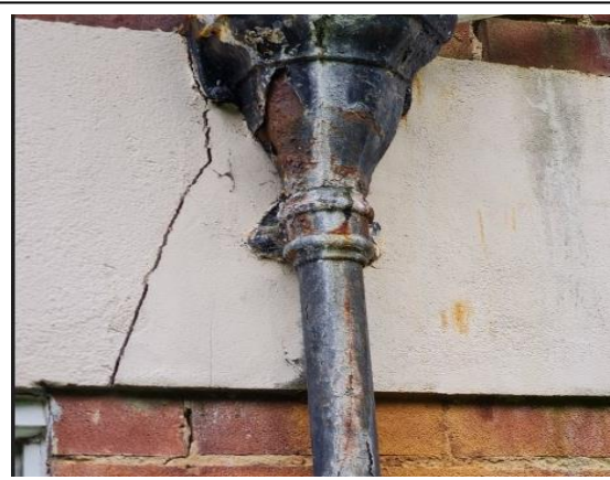
Photo 21: Rear Elevation – Cracking above Ground Floor Middle Window-
