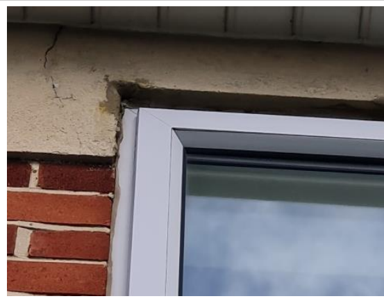
Photo 19: Cracking above First Floor Left Window
