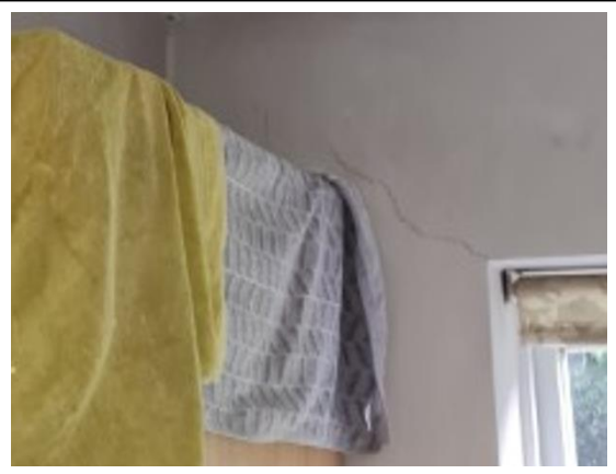
Photo 11: Flat 19 – Kitchen - Cracking Above LHS of Window
