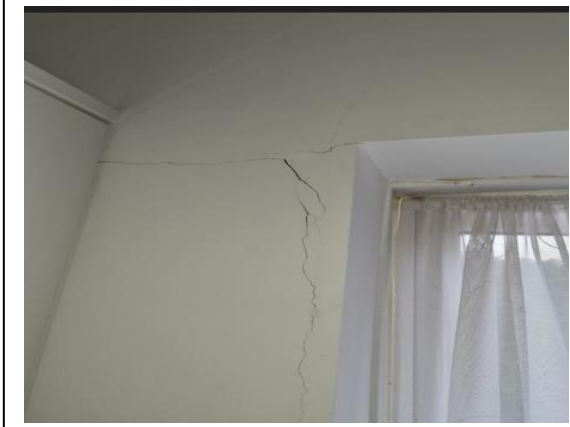
Photo 2: Flat 20 – Kitchen - Cracking to LHS of Window
