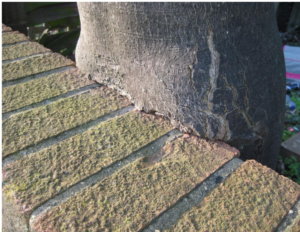
Image 2 – In places trees are in direct contact with the boundary wall and these trees should be considered for removal on health and safety grounds.
