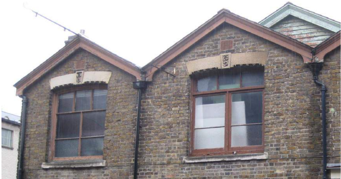
Figure 21: Lintels to the front façade have dropped slightly and are to be made good.
