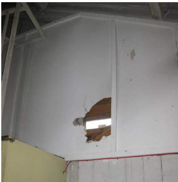
Figure 16: Hole present through roof gable. The roof covering is likely to be in a poor condition and require replacement. The hole will have let water into the structure.
