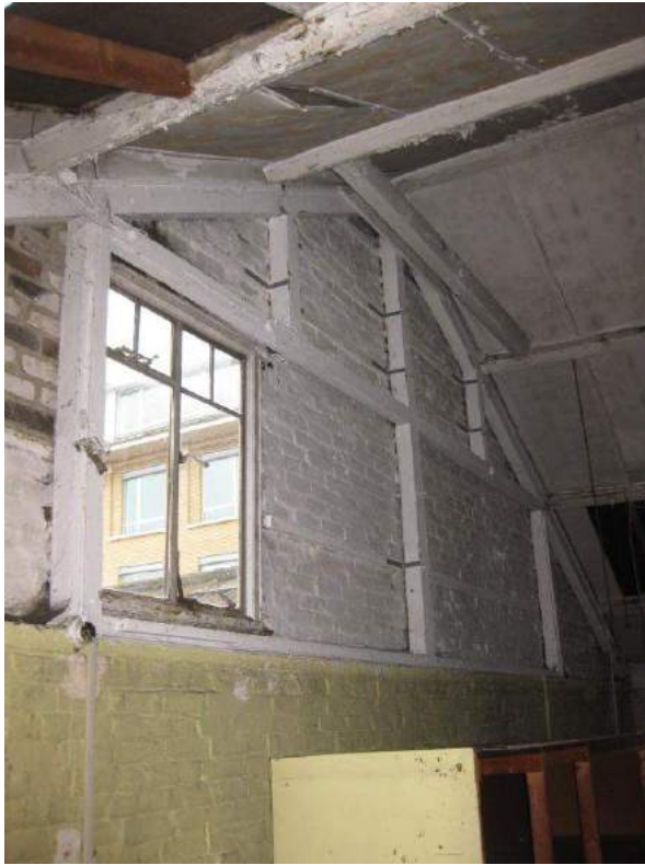
Figure 17: Roof gable next to the 1960s warehouse. At high level the thickness of the wall reduces to half a brick thick which is very thin. It appears that the timber frame on the inside face provides lateral restraint to the wall.
