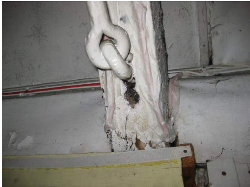
Figure 14: Detail of the steel tie fixing into the end of the timber rafter. The bolted connection shows evidence of rotating, slipping and failing the timber in bearing. This may have been exacerbated by the timber becoming wet.
