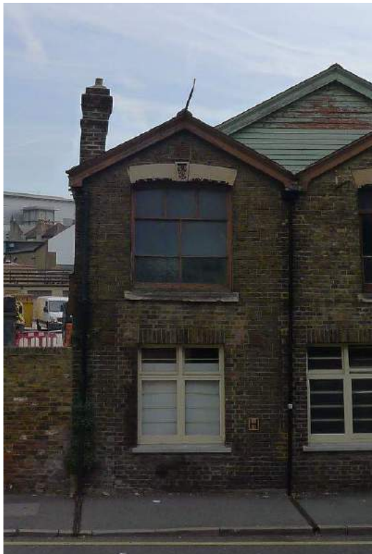
Figure 20: The chimney stack is leaning and potentially unstable.
