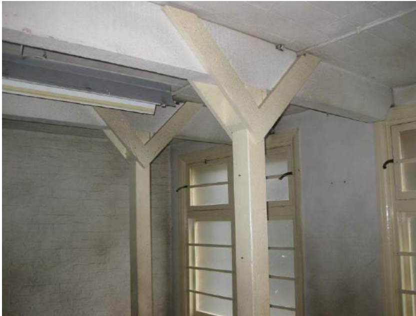
Figure 11: Support of the first floor structure behind the central bay. This structure is a poor quality modern alteration.
