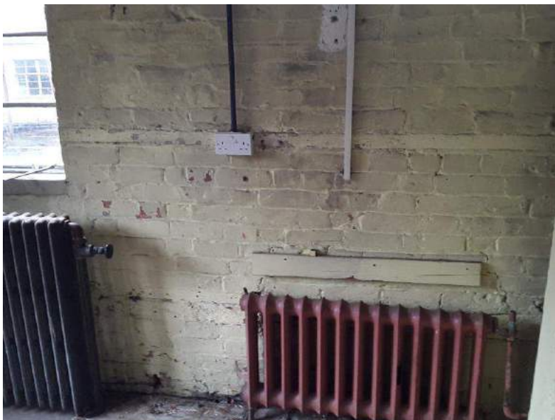
Figure 18: Timber is embedded into a number of masonry walls. It is recommended that the timber be removed and replaced with masonry to provide long term durability.
