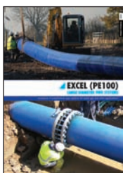
G0020 Large Diameter Pipe Systems
