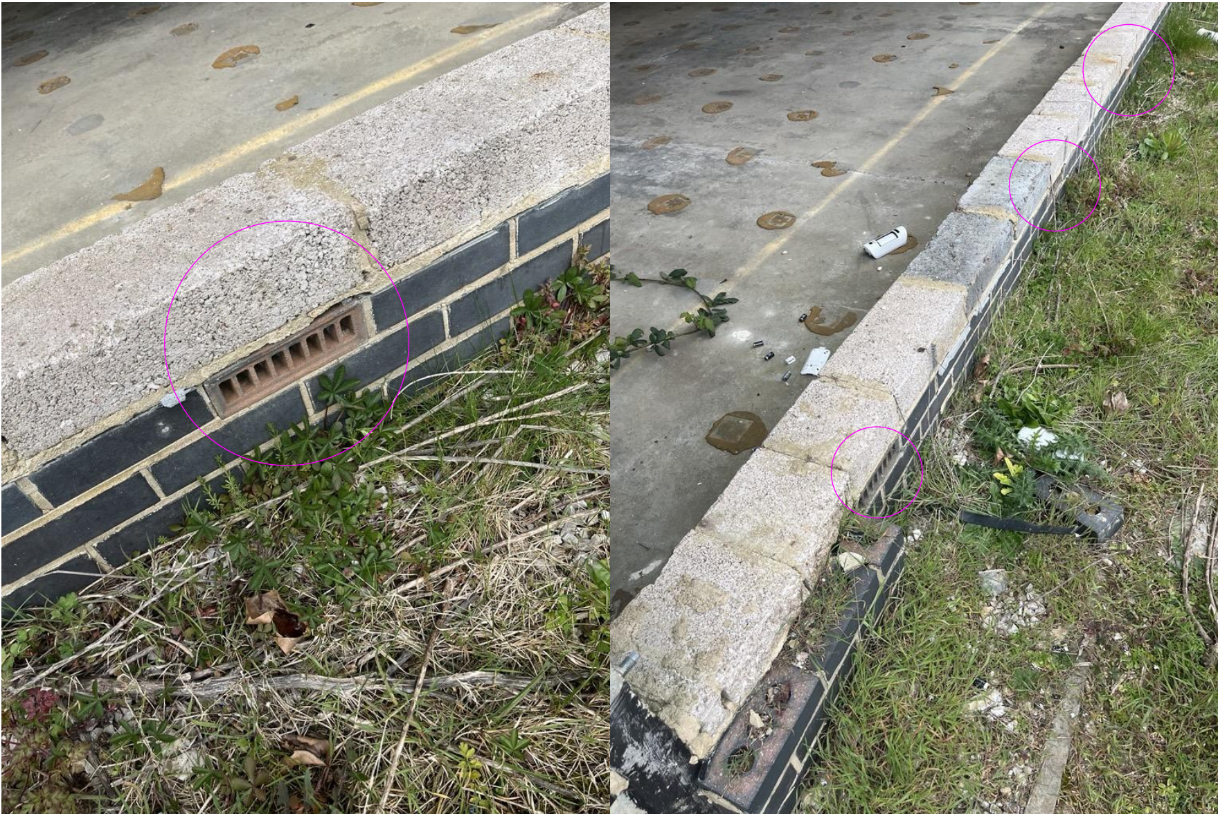
(SK)004_Existing Telescopic Vent Image
