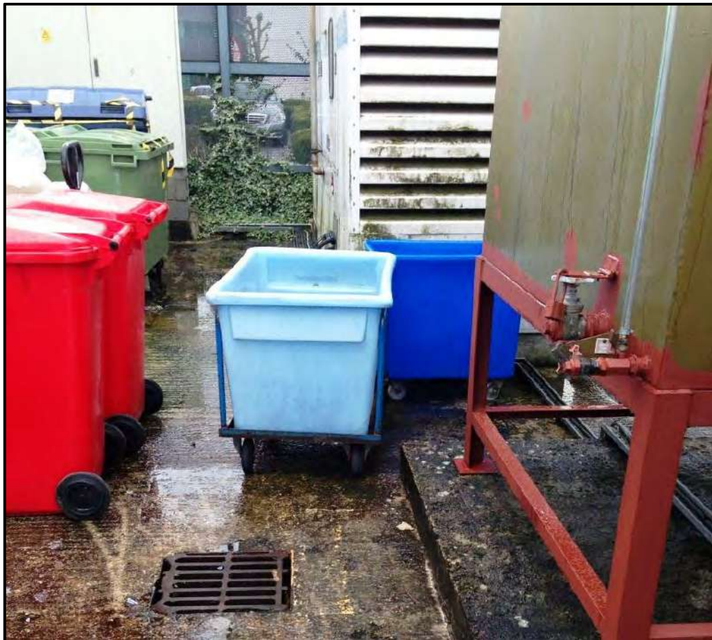
PLATE 2: 3,630 LITRE DOUBLE SKINNED DIESEL AST LOCATED ADJACENT TO A DRAIN, WITHIN AN ENCLOSURE TO THE SOUTH OF THE MULTI-STOREY CAR PARK.
