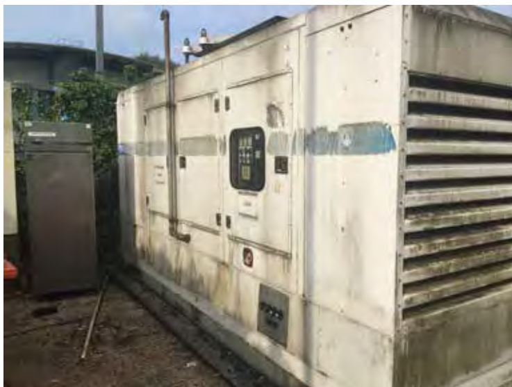
Back-up generator within enclosure in the centre of the Site
