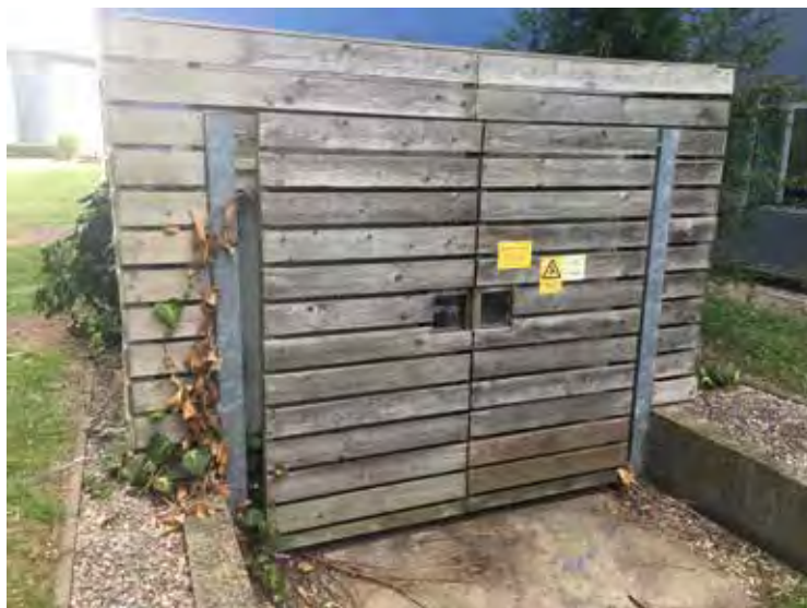
Self-contained electrical substation adjacent to Riverview House
