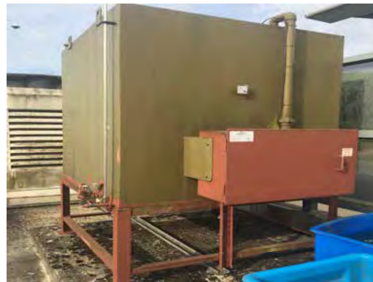
3,630-litre diesel AST used for adjacent back-up generator
