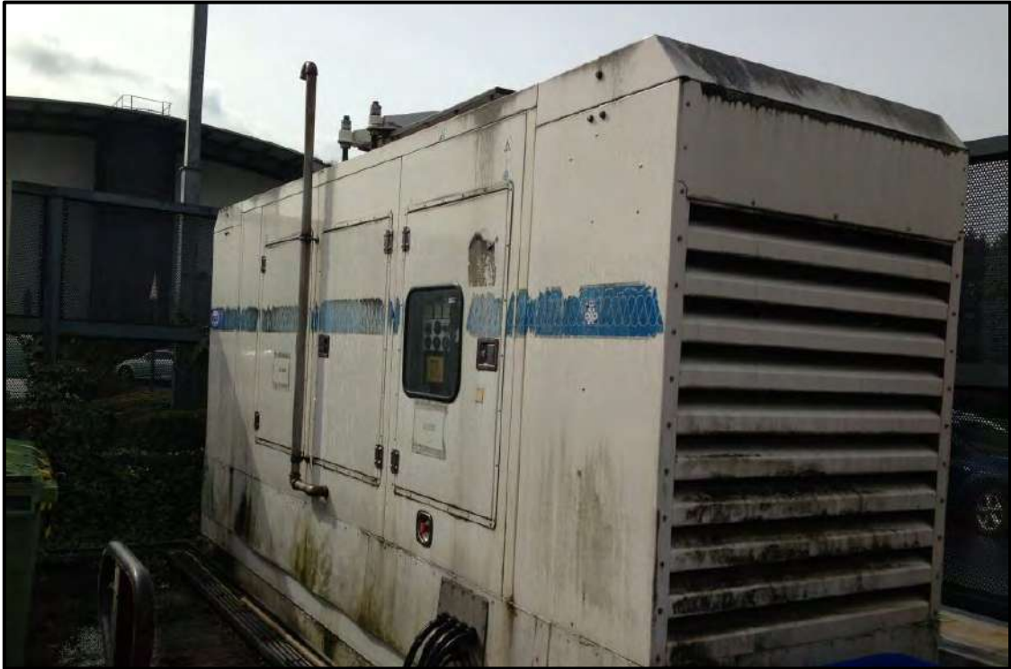
PLATE 3: BACK-UP GENERATOR LOCATED ADJACENT TO THE DIESEL AST ON-SITE
