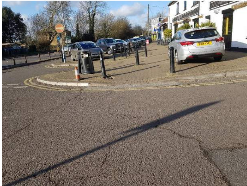
Photo 6 – No Tactile Paving on Oxford Road (Parade of Shops – Site Boundary) (L7)
