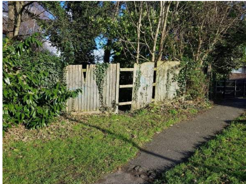
Photo 8 – Poor Maintenance on Oxford Road (Parade of Shops – Oakside North) (L8)
