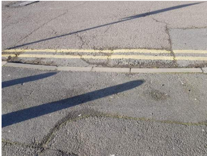
Photo 1 – Kerbs without Tactile Paving (L6)
