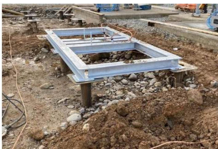
Examples of mini piles with ground beam constructions; reinforced concrete and a structural steel example.
