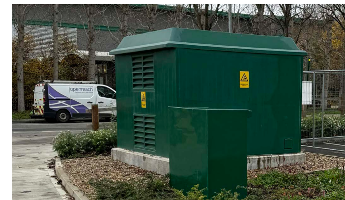
Existing RMU & Transformer
