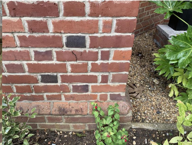
Stepped crack below Lounge window
