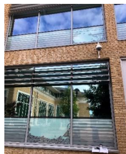
Figure 9. 4 th Failed Manifestation
