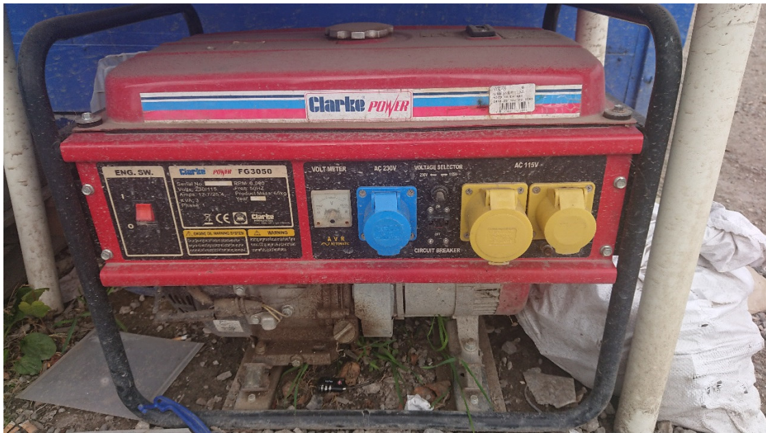
Figure 4: Photo of the Standby Generator In-Situ
