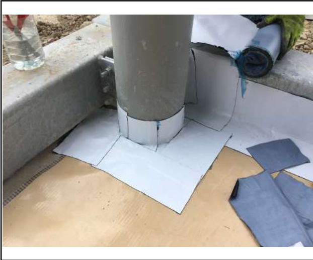
Pipe work in awkward position
