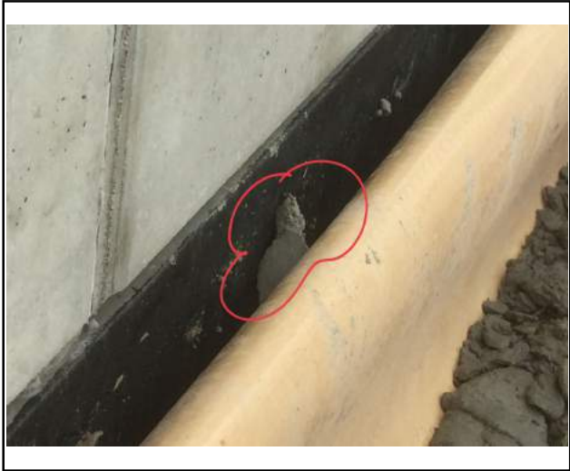
Debris trapped requiring removal
