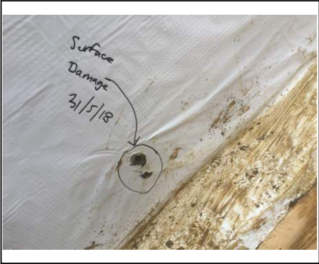
Damage to GRSA Membrane - Lift Pit
