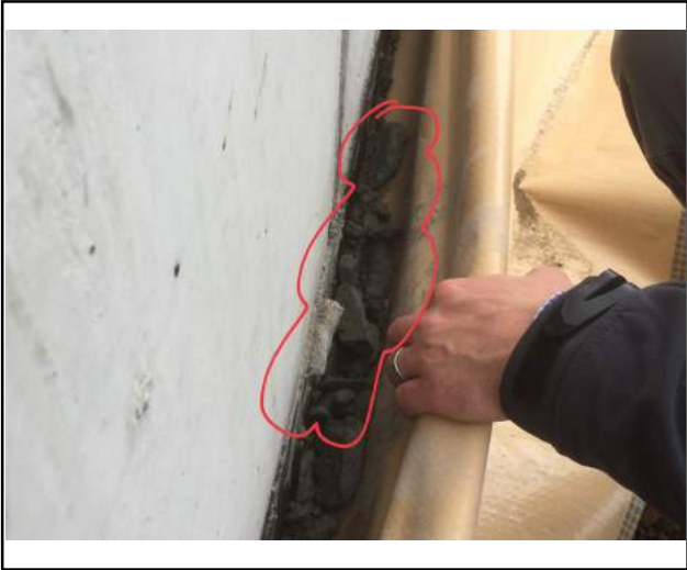
Debris trapped requiring removal
