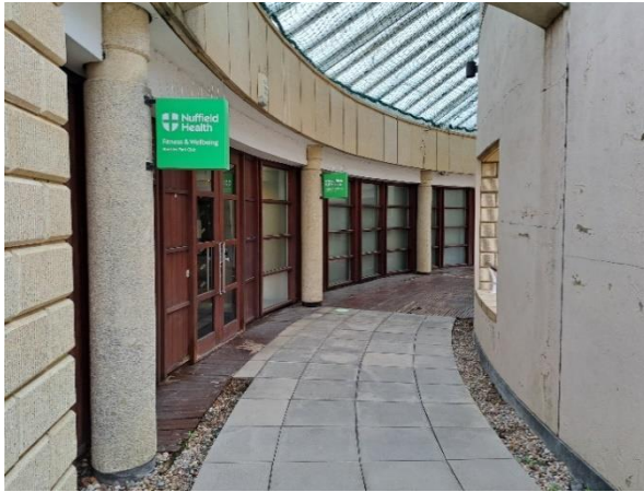
Figure 3.5: The Arena – first floor Rotunda walkway with deteriorating patent glazing.
