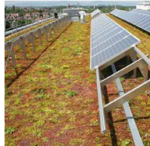
Roof mounted PV panels
