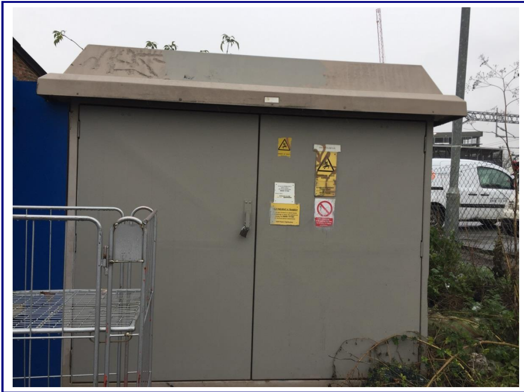
Photo 3: Electricity sub-station located to the west of the site.
