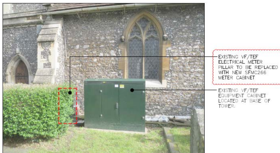
EXISTING EXTERNAL EQUIPMENT LOCATION
