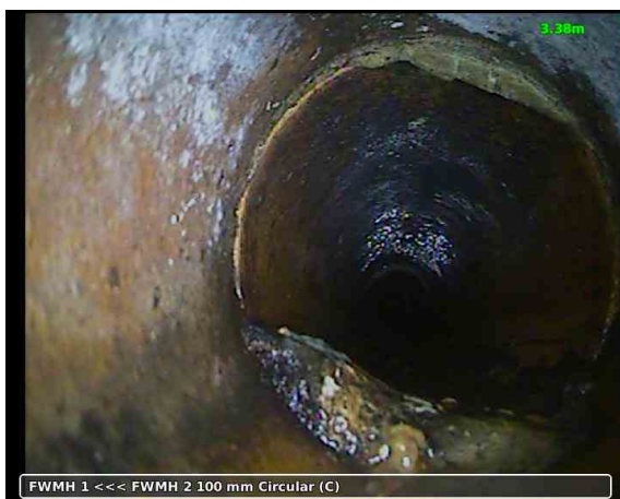
20190615-105947-snap0002.jpg, 00:00:55, 3.38 m Attached deposits, encrustation, from 05 to 07 o'clock, 15 % cross-sectional area loss
