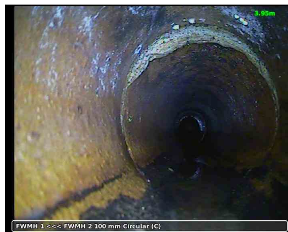
20190615-105947-snap0003.jpg, 00:01:20, 3.95 m Attached deposits, encrustation, from 09 to 03 o'clock, 5 % cross-sectional area loss
