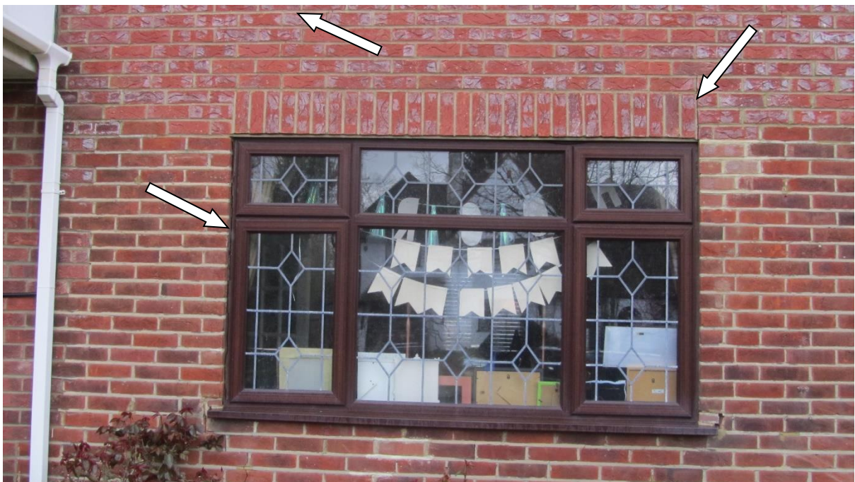
PHOTOGRAPH NO. 4 - Brickwork cracking and window displacement on the front elevation of No. 2 Ebury Close (arrowed)
