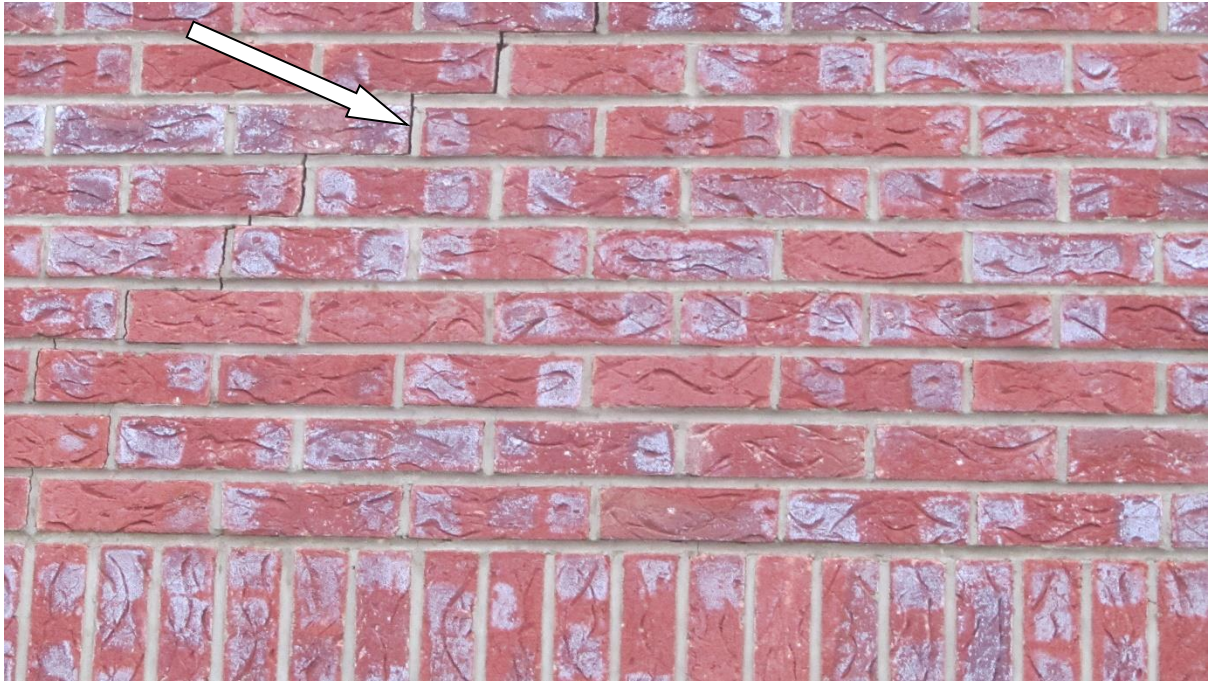
PHOTOGRAPH NO. 3 - Stepped brickwork cracking on the front, southern elevation near to the southeast corner (arrowed)
