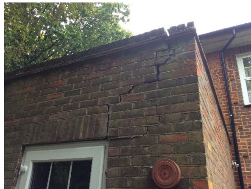
Cracking to Rear Left-Hand Corner
