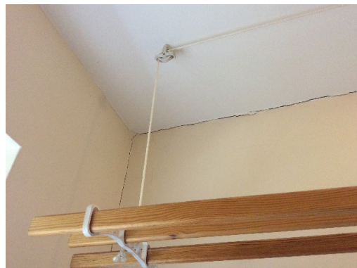
Cracking to Utility Room
