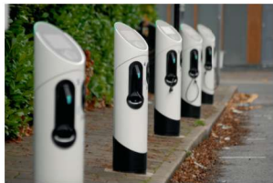
2 EV Charger Point
