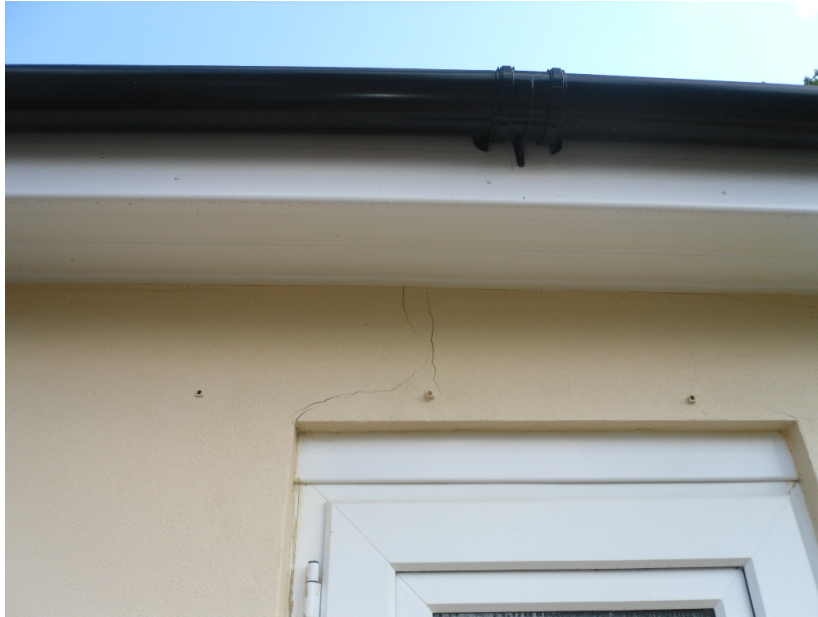
Cracking above utility room door
