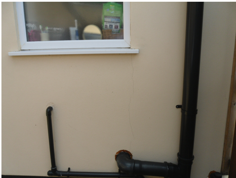
Hairline crack below bathroom window
