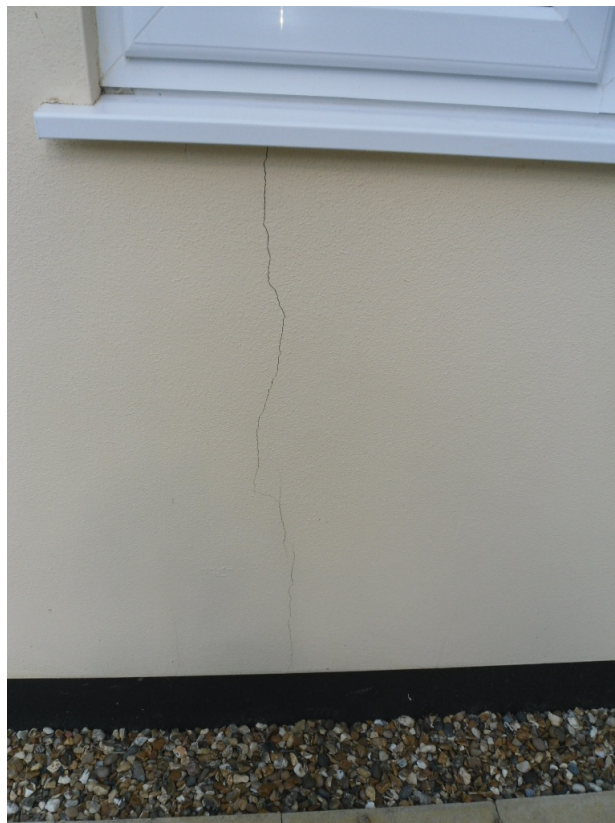
Cracking below kitchen window
