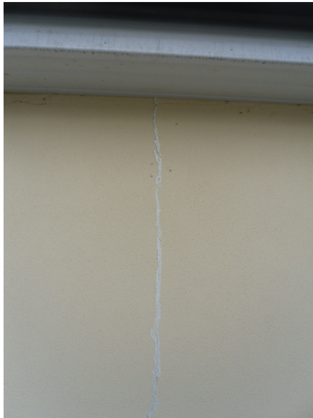
Cracking to extension/original house junction
