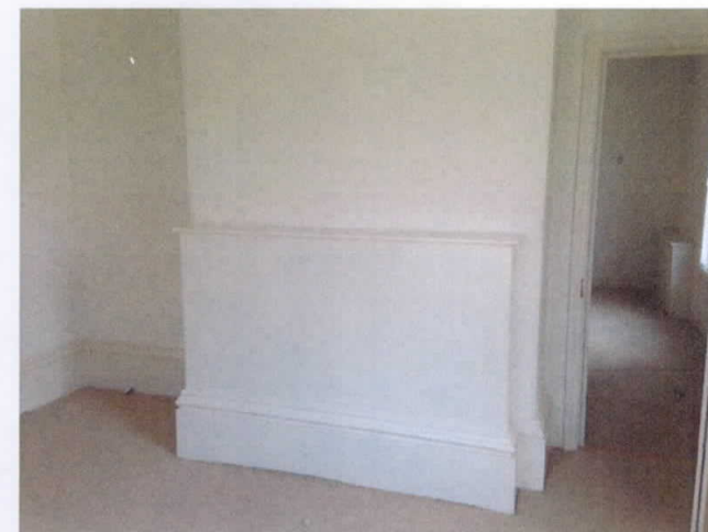
Plate 14: Typical room with blocked chimney
