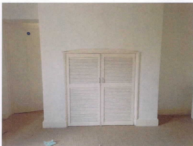
Plate 15: Typical room with blocked chimney
