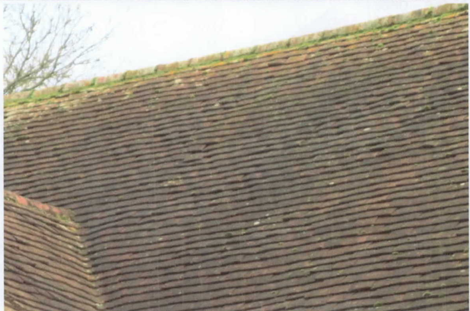
Plate 11 – Building 3 Office Barn View of roof (general) showing extensive gaps under tiles
