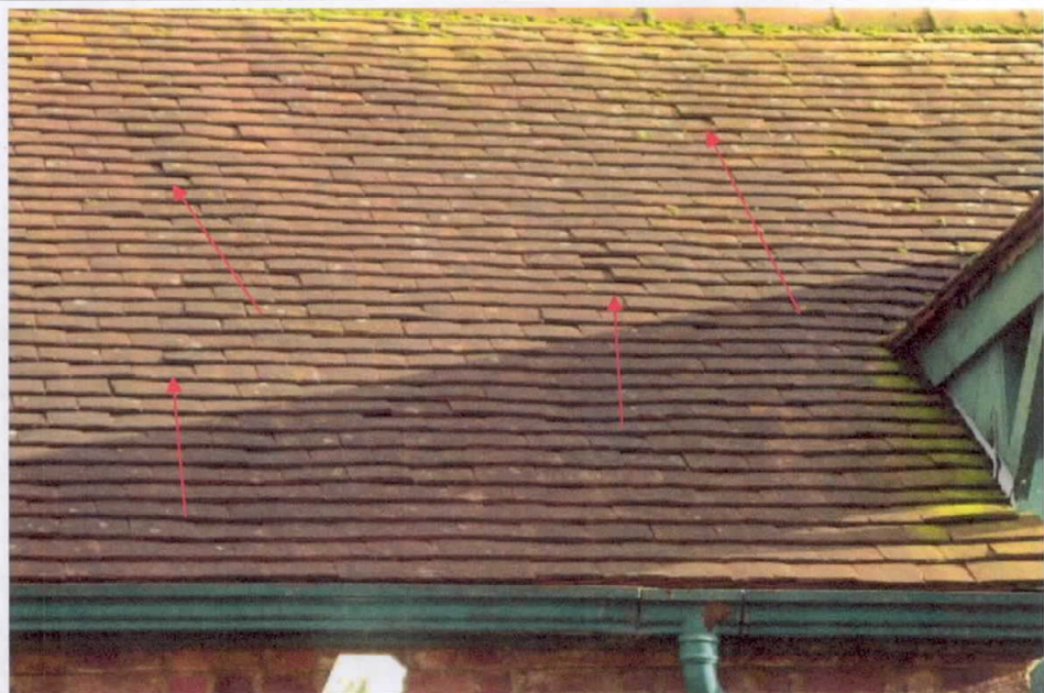
Plate 7 – View of roof covering of Building 2 – Former Stable Block showing extensive gaps that could be used by bats
