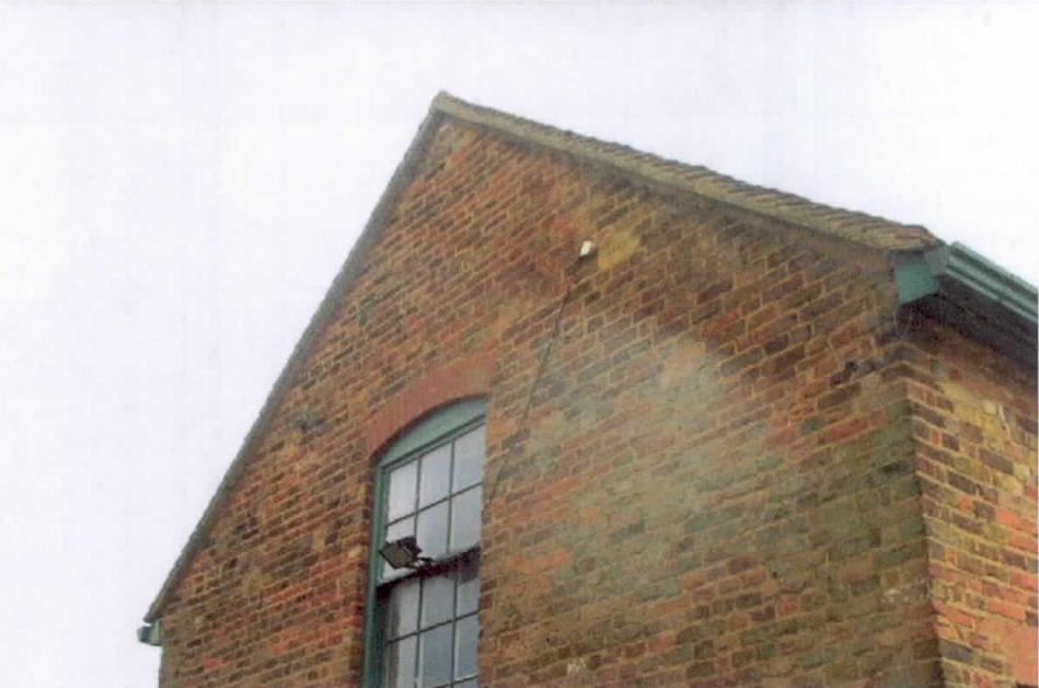
Plate 4 – Building 2 – Former Stable Block – North facing Gable end showing condition of pointing.
