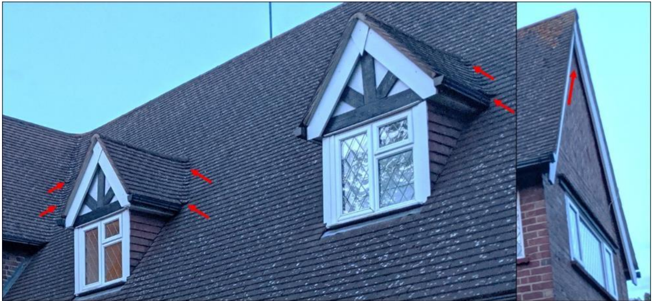
Photograph 1: Showing gaps beneath valley tiles and barge board on the house.
