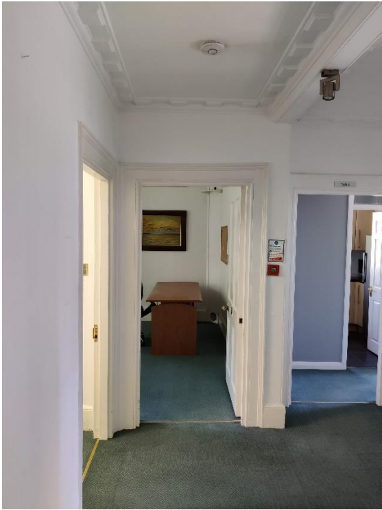
Distortion to first floor front left side door.
