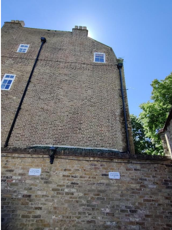
Blocked rain water downpipe.
