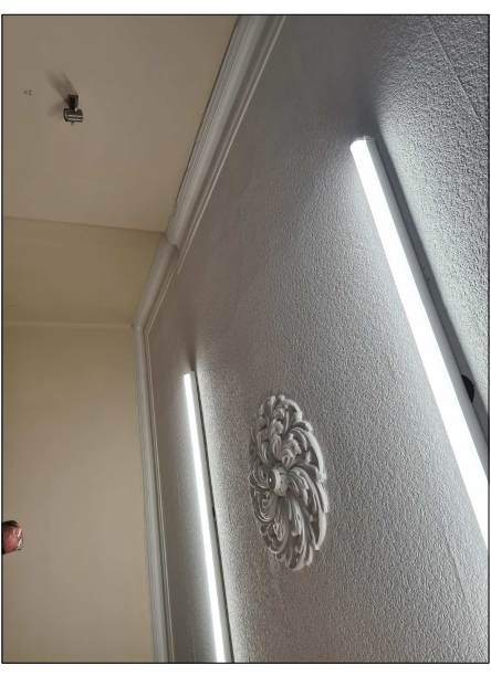
Minor plaster cracks to be rubbed down, spot filled & redecorated - Ceiling rose retained.
