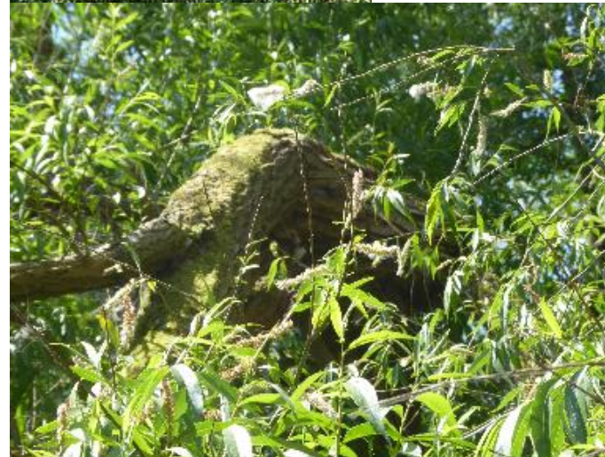
T15 Willow sp - mature Main stem cracked at c.8m (leaning east). Splits and potential cavities present around cracked section. Moderate potential
