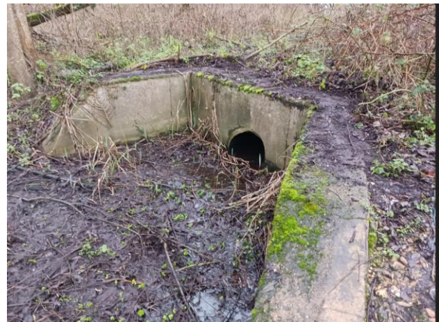
(b) Pipe outlet
