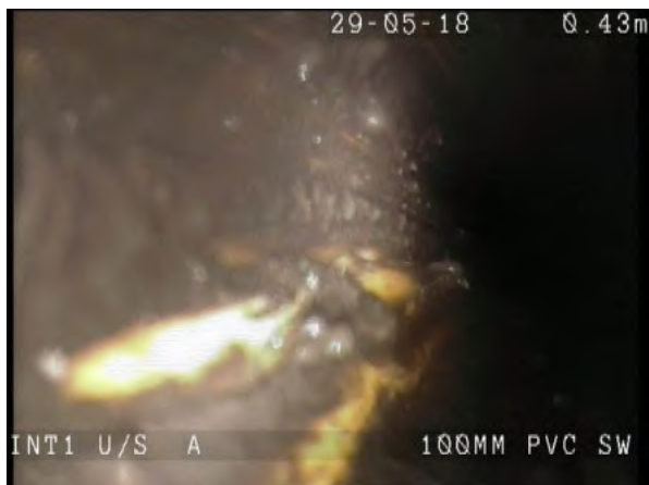
A_INT1X_d93bc85b-68b5-4cbd-a036-2f44e01cce6d_20180604_112539_134.jpg, 00:00:08, 0.30m Settled deposits, fine, 5% cross-sectional area loss
