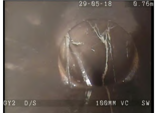
GY2X_33c5c1ea-f169-4d8f-ada0-a495ecdef433_20180604_114148_482.jpg, 00:00:12, 0.80m Joint displaced, medium
