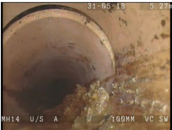
A_MH14X_f734058e-39ba-499b-9f6f-974fac535ce5_20180604_143727_323.jpg, 00:00:38, 5.30m Joint displaced, medium
