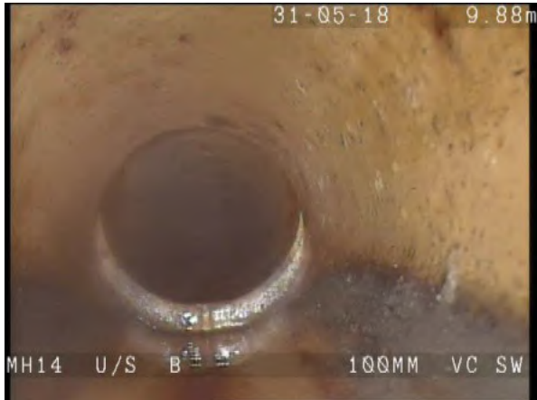
B_MH14X_f80fcc4a-b6ef-4fc9-a41e-e90103d837d1_20180604_145211_035.jpg, 00:01:13, 10.00m Joint displaced, medium
