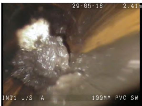
A_INT1X_e7e7eead-7a53-40b7-88a5-a5bca6dd5703_20180604_112635_734.jpg, 00:00:23, 2.50m Settled deposits, fine, 40% cross-sectional area loss
