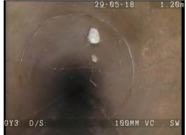
GY3X_50057357-3fb3-43e8-84e6-5fc63ff7c92e_20180604_115348_849.jpg, 00:00:13, 1.30m Crack, circumferential from 12 o'clock to 12 o'clock
