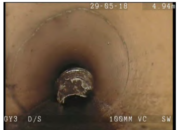
GY3X_b9039a48-1108-4694-bd18-1360eff10592_20180604_115439_085.jpg, 00:00:31, 5.00m Crack, circumferential from 7 o'clock to 5 o'clock
