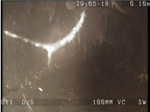
GY1X_4ae48c69-bb7e-4f0a-8a19-bf8cd0d8e4c5_20180604_113150_073.jpg, 00:00:06, 0.10m Settled deposits, fine, 5% cross-sectional area loss, start
