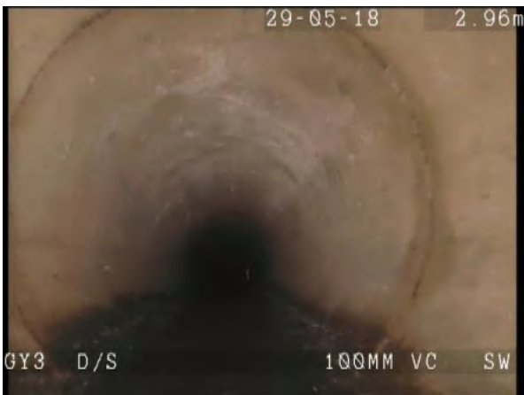
GY3X_f5782e97-a6ba-4fec-a11c-89e9b0a02103_20180604_115415_309.jpg, 00:00:23, 3.00m Crack, circumferential from 7 o'clock to 5 o'clock
