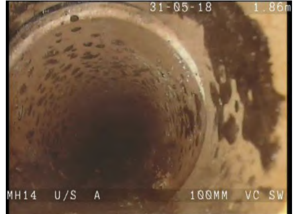
A_MH14X_0ebe5ef9-0fe6-42d8-a01f-5de9df510e83_20180604_143440_621.jpg, 00:00:16, 1.90m Joint displaced, medium
