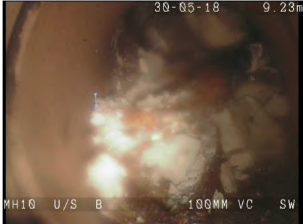
B_MH10X_4d6fb09f-78bf-47cb-b3e9-59aa1e942ddd_20180604_122311_591.jpg, 00:00:54, 9.30m Settled deposits, coarse, 90% cross-sectional area loss
