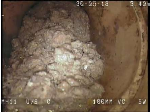
C_MH11X_2567db29-1375-41da-92e6-dec86a3494df_20180604_131952_395.jpg, 00:00:29, 3.40m Settled deposits, coarse, 95% cross-sectional area loss
