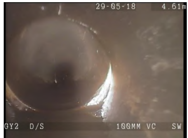
GY2X_a79ea17b-9a1f-4af5-83d4-555353067472_20180604_114230_449.jpg, 00:00:34, 4.70m Joint displaced, medium
