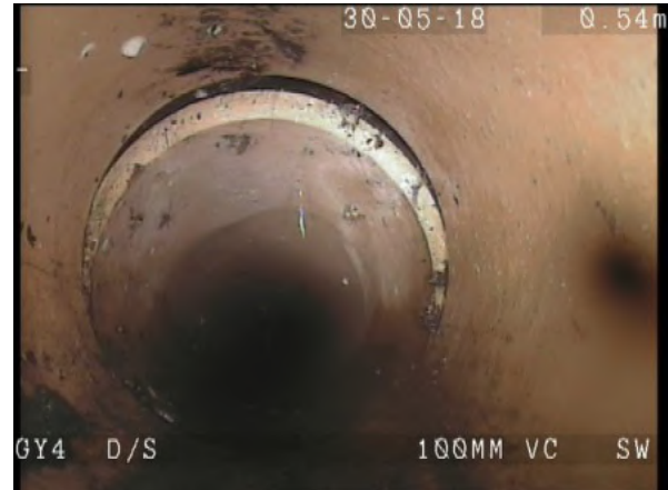
GY4X_fb7ebc75-bacb-4bc7-9aa2-9c46b27d4ab2_20180604_132856_232.jpg, 00:00:18, 0.60m Joint displaced, medium
