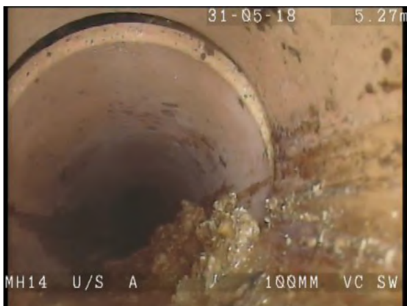
A_MH14X_f734058e-39ba-499b-9f6f-974fac535ce5_20180604_143727_323.jpg, 00:00:38, 5.30m Joint displaced, medium
