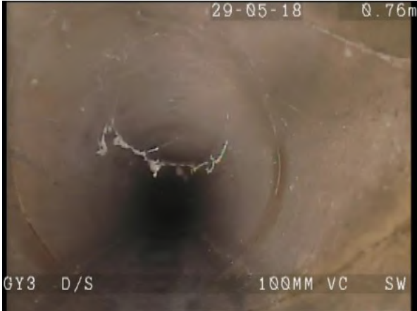
GY3X_dd9d2f66-7a16-4d3e-a03f-82c0c425fc5c_20180604_115332_276.jpg, 00:00:10, 0.80m Crack, circumferential from 12 o'clock to 12 o'clock
