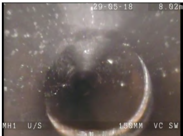
MH3X_a3ddf67a-6157-40fe-801c-e0e08bedef87_20180604_105126_505.jpg, 00:00:36, 8.10m Joint displaced, medium
