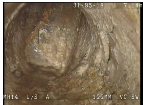
A_MH14X_9e96a233-ed1c-48e5-94ed-759369fd6198_20180604_143909_323.jpg, 00:00:52, 7.20m Other obstacles from 5 o'clock to 7 o'clock, 20% cross-sectional area loss
