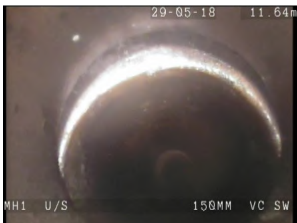
MH3X_d36944c7-39db-467e-8472-70c44a59c664_20180604_105151_525.jpg, 00:00:48, 11.60m Joint displaced, medium
