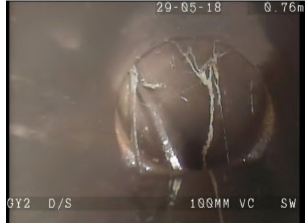
GY2X_33c5c1ea-f169-4d8f-ada0-a495ecdef433_20180604_114148_482.jpg, 00:00:12, 0.80m Joint displaced, medium
