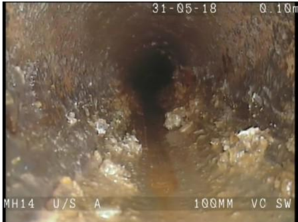
A_MH14X_04528b0a-7455-46eb-b22f-35010d4167e5_20180604_143517_428.jpg, 00:00:05, 0.10m Attached deposits, grease from 3 o'clock to 8 o'clock, 5% cross-sectional area loss
