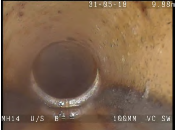
B_MH14X_f80fcc4a-b6ef-4fc9-a41e-e90103d837d1_20180604_145211_035.jpg, 00:01:13, 10.00m Joint displaced, medium
