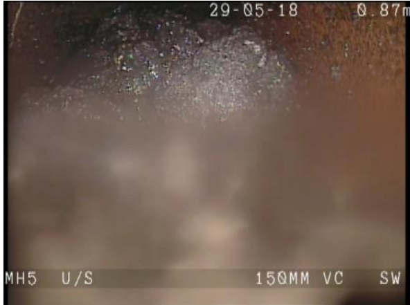
MH4X_43c76f17-273d-43f7-9a21-59457ef01918_20180604_11 5830_834.jpg, 00:00:25, 1.00m Settled deposits, fine, 80% cross-sectional area loss
