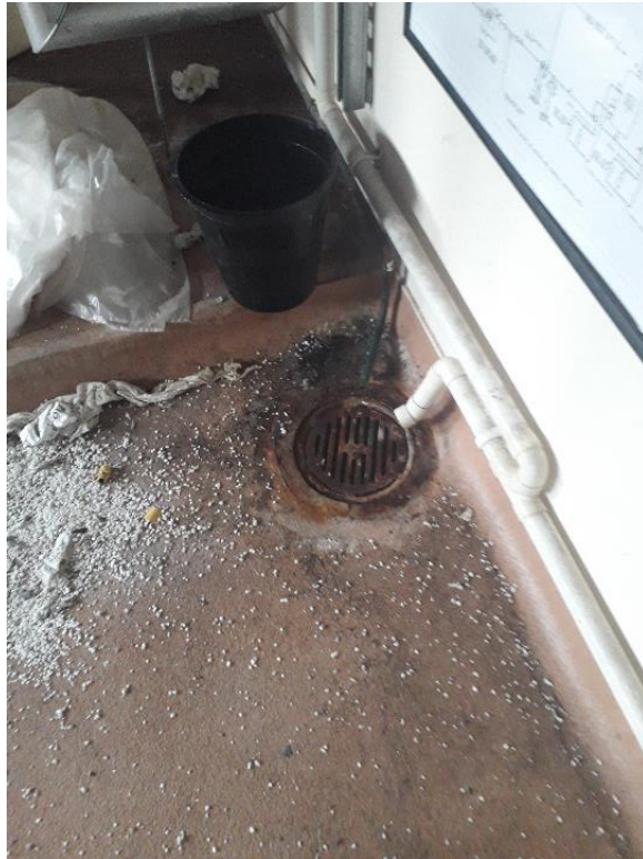
Photograph 13: Staining noted on the floor within plant room
