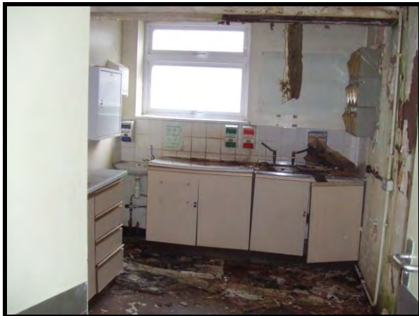
Plate 03 – Example of room in disrepair
