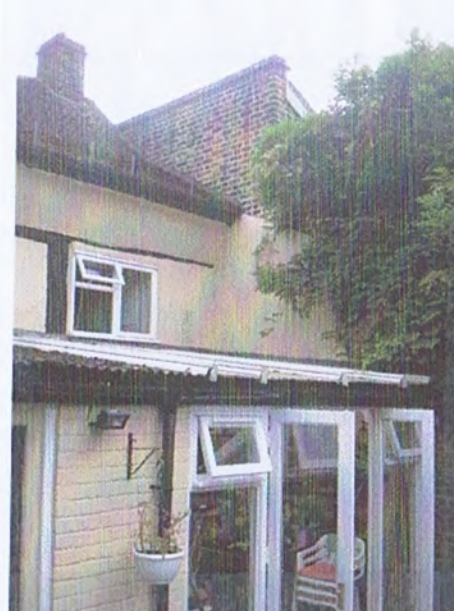
asbestos-cement corrugated roof (proposed replaced)
