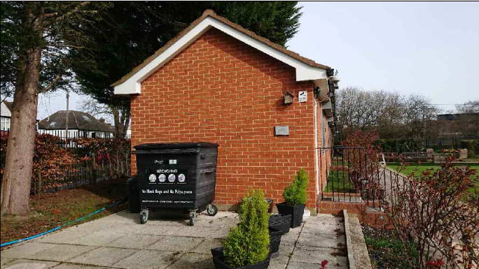
VIEW OF FUSE BOX AND WATER TANK
