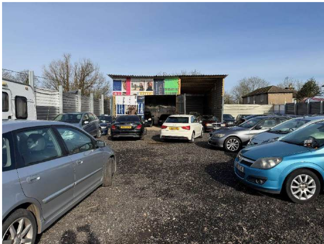
Photograph 3: View of temporary structure to west of derelict residential property, facing north.
