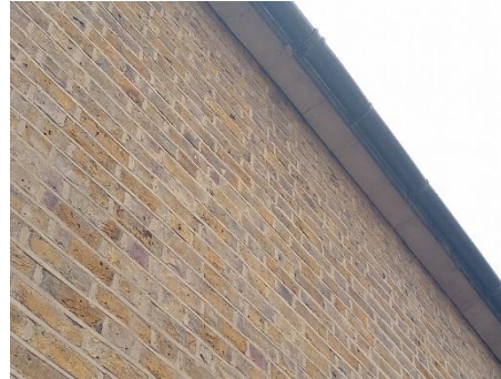
Very minor crevice at soffit board
