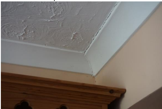
Kitchen - Ceiling junction separation
