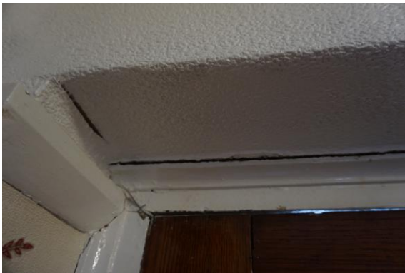
Hall - Separation to door frame
