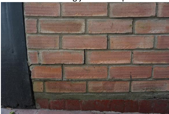
Right Elevation Porch - Stepped crack
