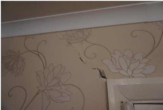
Lounge - Diagonal crack above door
