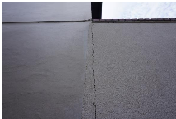
Right Elevation - Vertical crack at extension junction
