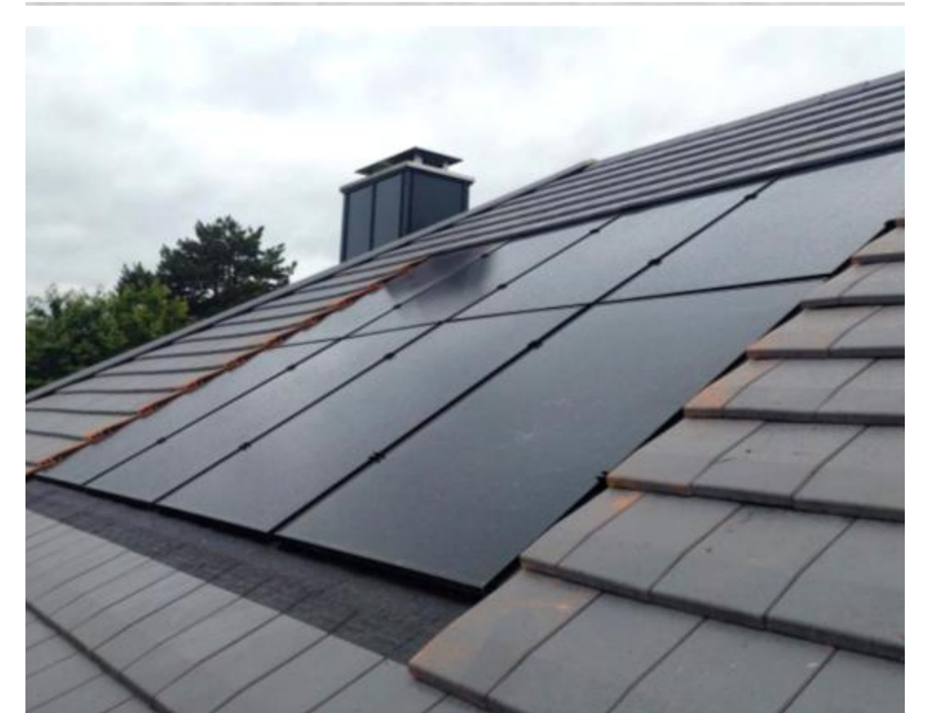
4 In-Roof Photovoltaic Panels
